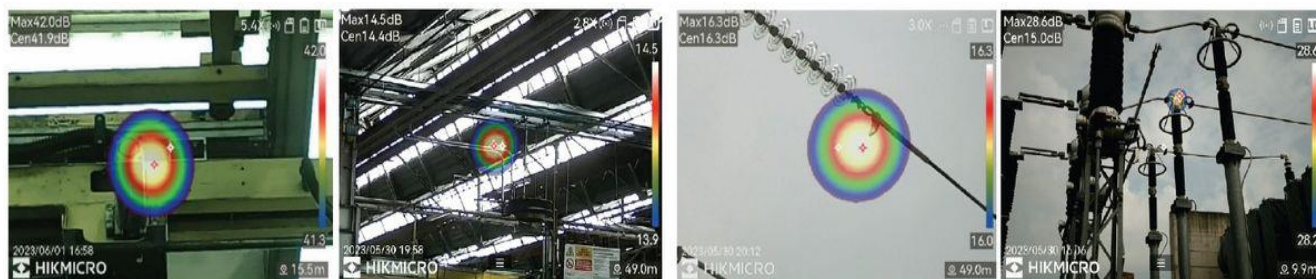
Gas Leak Detection
