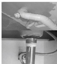
Water Supply Pipe Leakage/ Water Pipe Leakage
