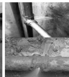
Fire Sprinkler System
